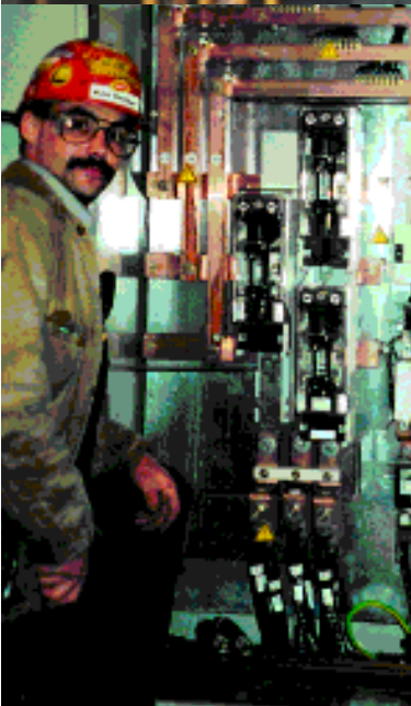
IBEW Local 48 marine electrician Ken Oerther, a recently graduated apprentice, inspects a motor control center on the Esperanza , a 124-megawatt power barge project at the Portland Ship Repair Yard.
